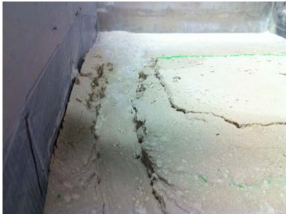
Fig. 4. The levee with 87.5cm length and 39.5cm width failed in centrifuge test; water flow = 0.56 lit/min, g = 20
